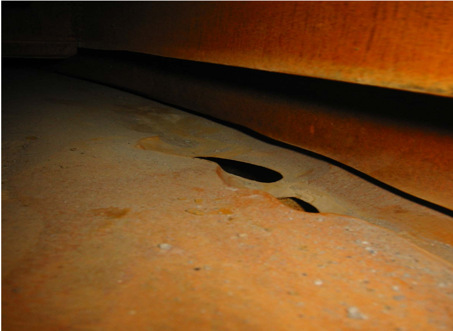
Cold End Sector Plate Erosion
